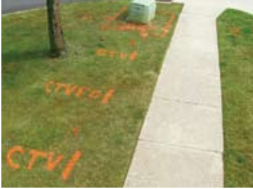
Example of cable TV pedestal, fiber optic, coax cable
